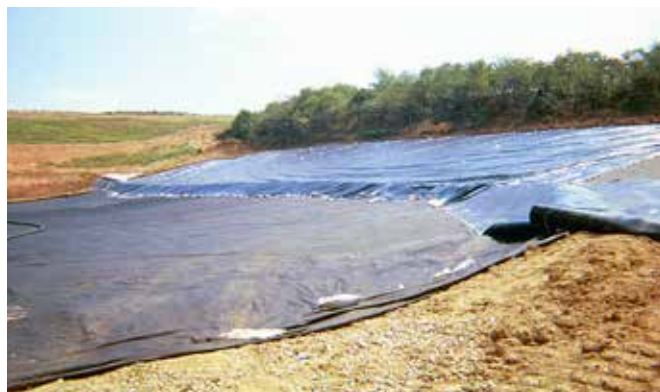
Interim Landfill Cover
