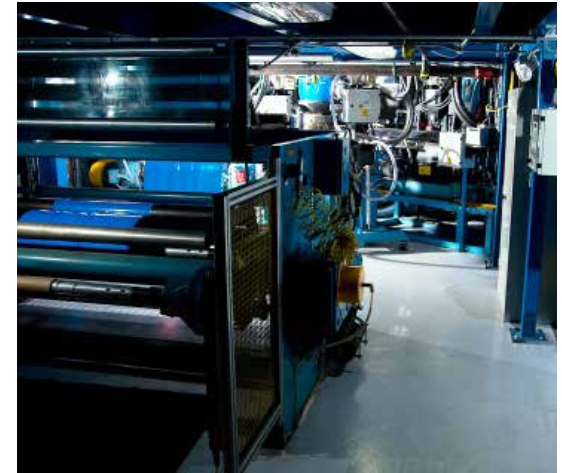
▶ View of the extrusion line winder section with a maximum roll capacity of 24" inch diameter.
