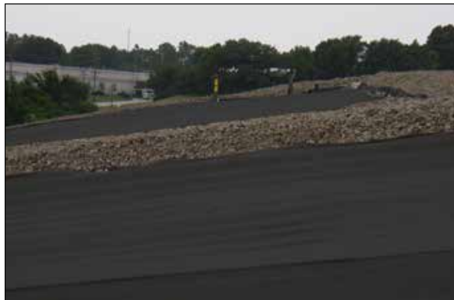
Landfill Odor Control Barrier
